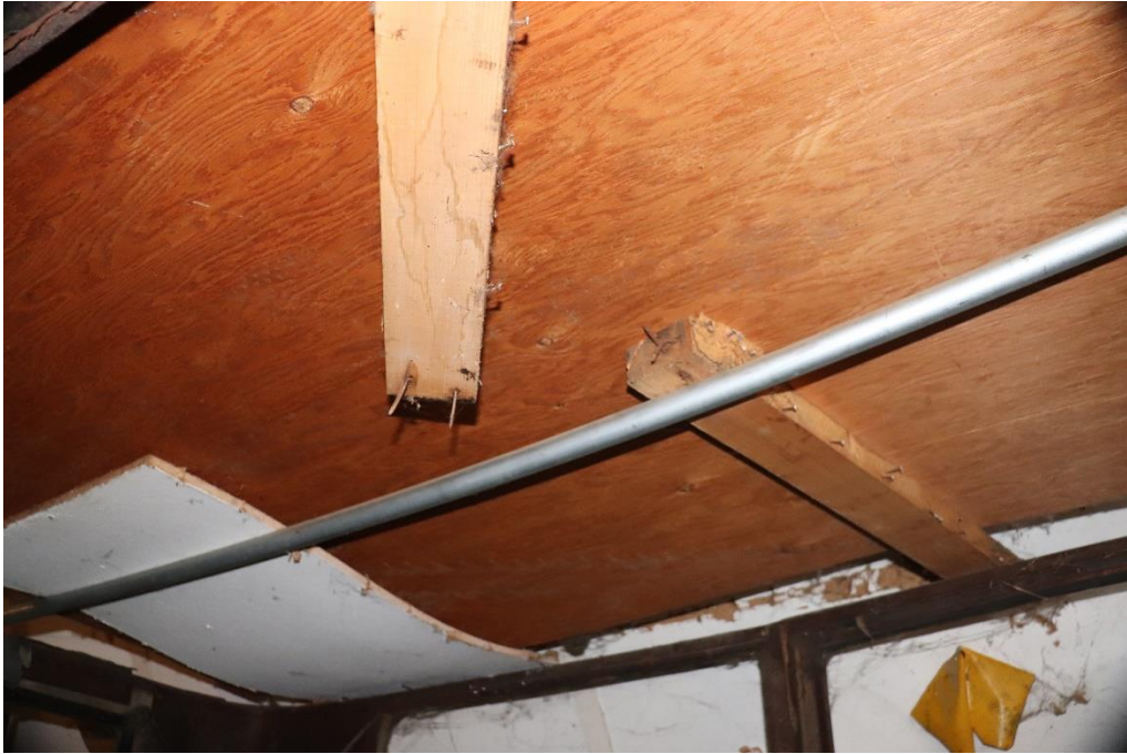
The roof insert is missing. The plywood seen is a shelf in place on the roof for storage purposes.
